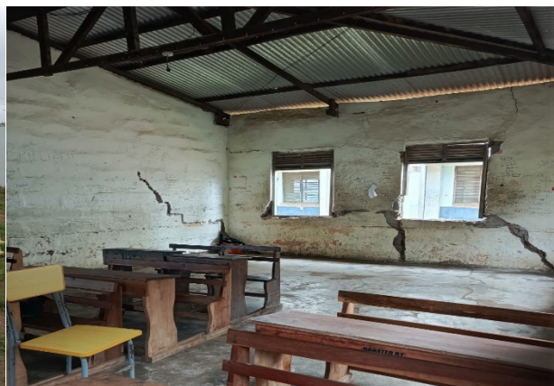
Classroom with deep cracks in wall at Teshie Presec.
