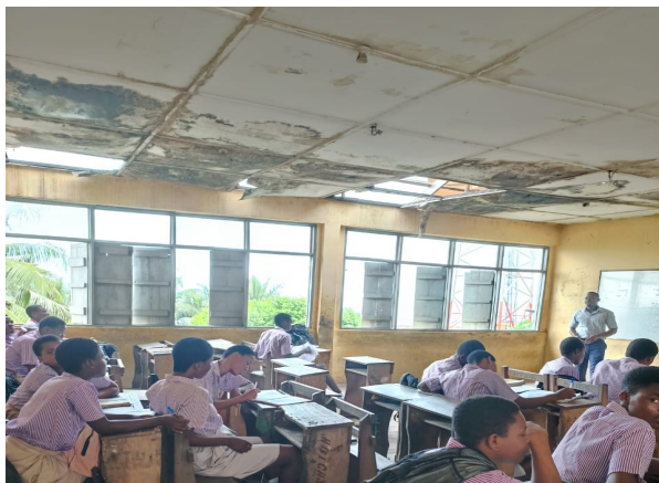
Ceiling with ripped off roof.
