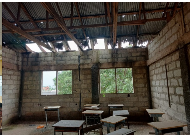
Classroom with torn roof at Presec-Teshie
