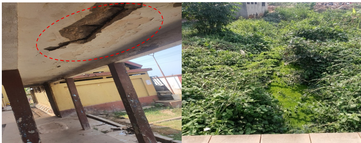
Deteriorating slab over a walkway at GSTS, Takoradi
