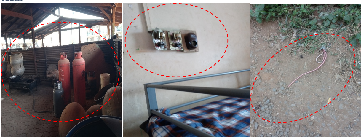
Gas cylinders close to burners at food preparation area, Oti Boateng SHS.
